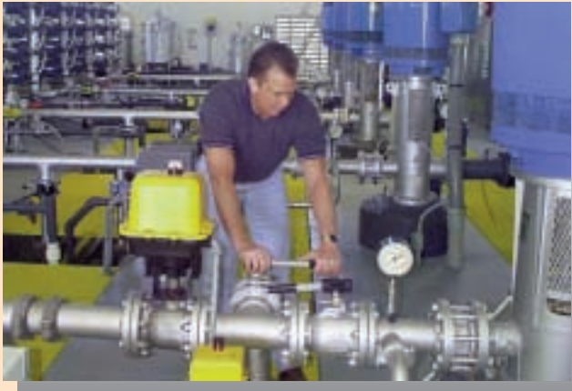
After filtering to remove the larger solids, the water passes through equipment where reverse osmosis is used to produce purified water.
